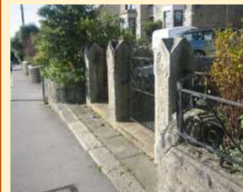
Dressed and carved granite piers bring quality to late Victorian villas on Higher Trevarthian Road
